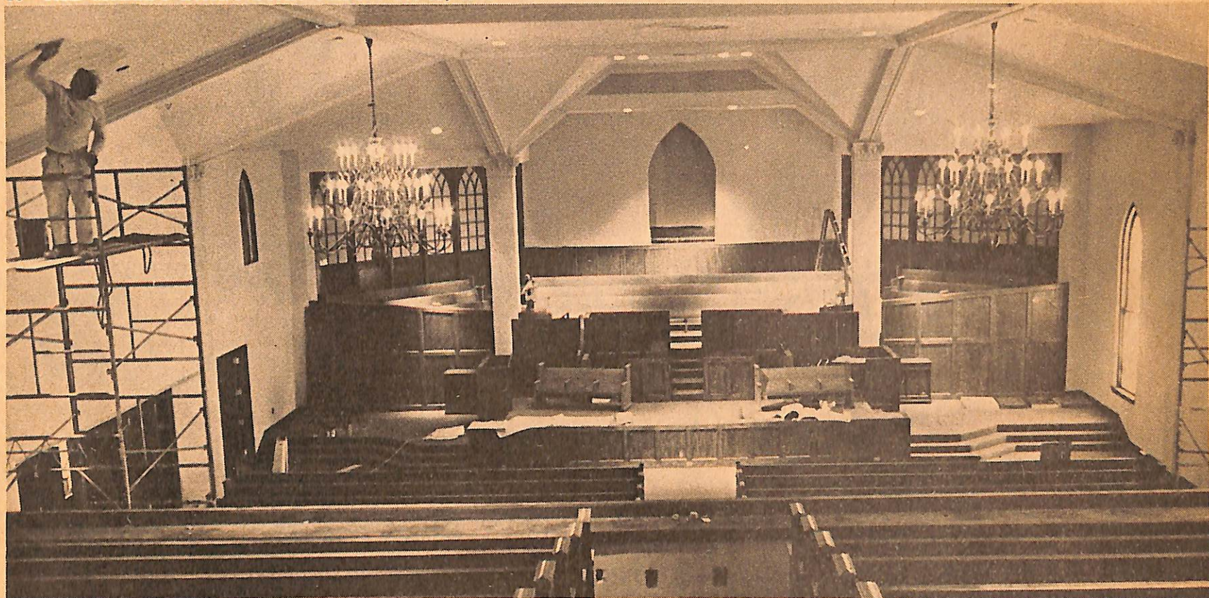
SANCTUARY READY — After a year and one-half of construction, the sanctuary of the First Baptist Church of Shelby is ready for regular Sunday services. The seating capacity of the rectangular sanctuary has been enlarged from 900 to 1,325. (Staff Photo by George Doggett)
