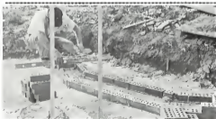
FIRST LAYER . . . Brickwork has progressed far beyond this stage on the Tower of Lights in the new entrance. Earl Harris is shown laying the foundation of the 30-foot tower.
